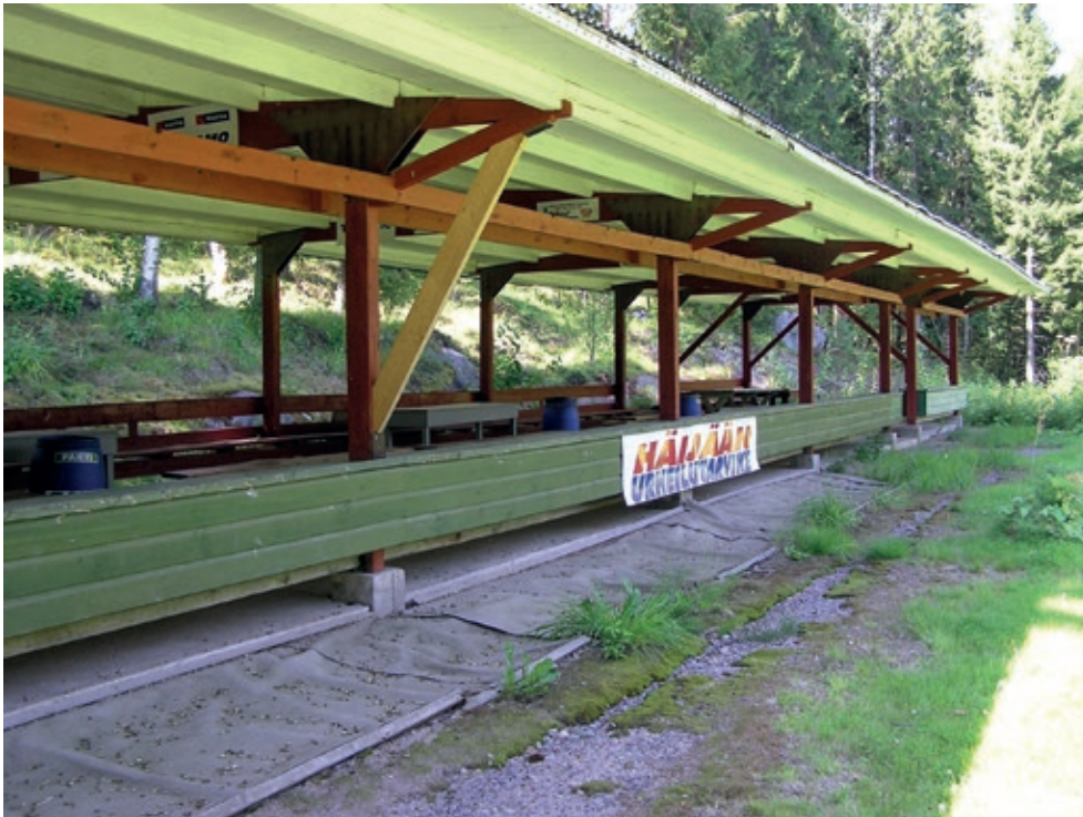
Figure 9.10. The open enclosure at the Nokia pistol range without noise prevention structures.
