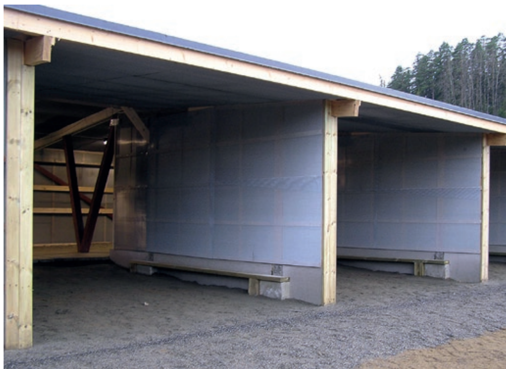
Figure 9.8. Enclosure with 4.6 m long noise-attenuating partitioning walls.
